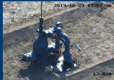
oil leakage identification
